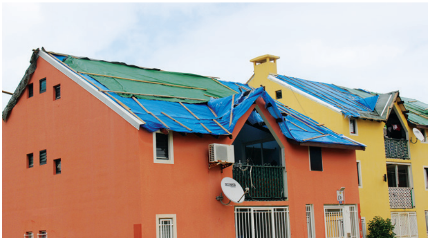
Figure 1: Damage to roofs
