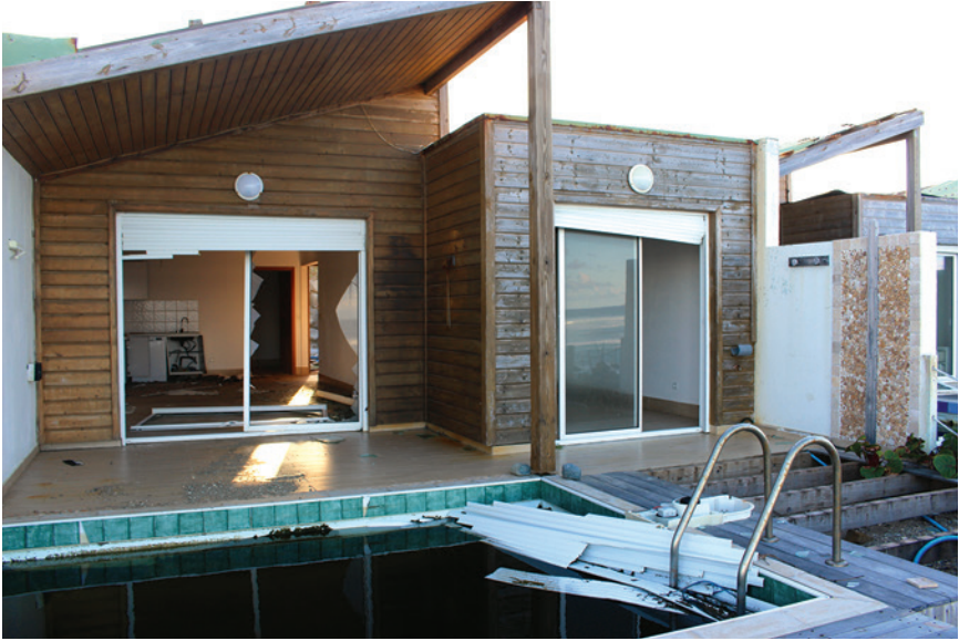
Figure 2: Damage to patio doors
