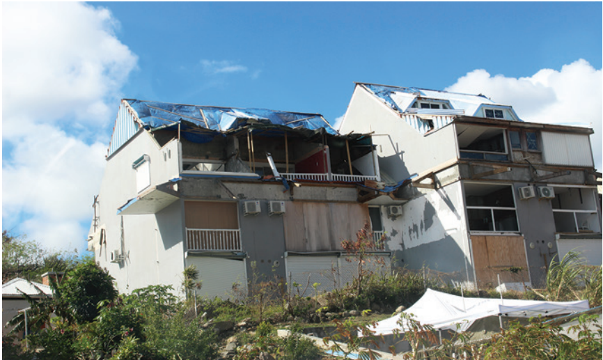
Figure 3: Damage to lighter sections of masonry buildings
