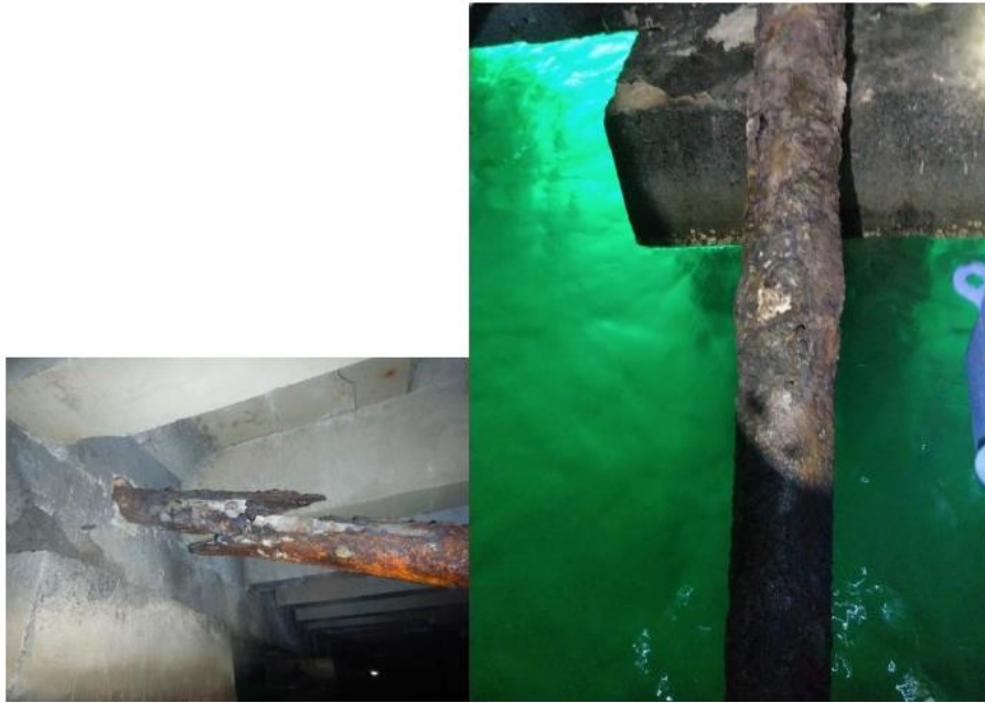
Figure 8 : Rupture de tirants, inspection de 2020(ACCOAST, AMAYA)
